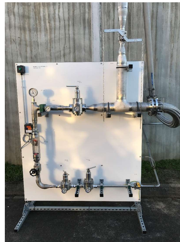
Manual control panel PO dosage
